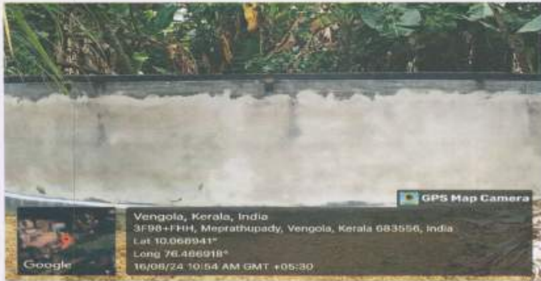
Rain Water Harvesting(Recharge Well)
