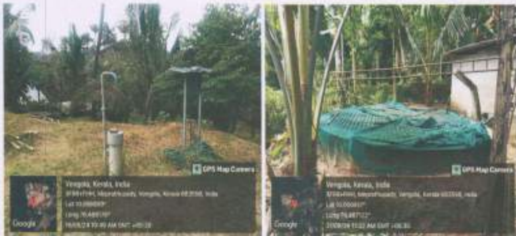
Ground Water System (Well & Bore well)
